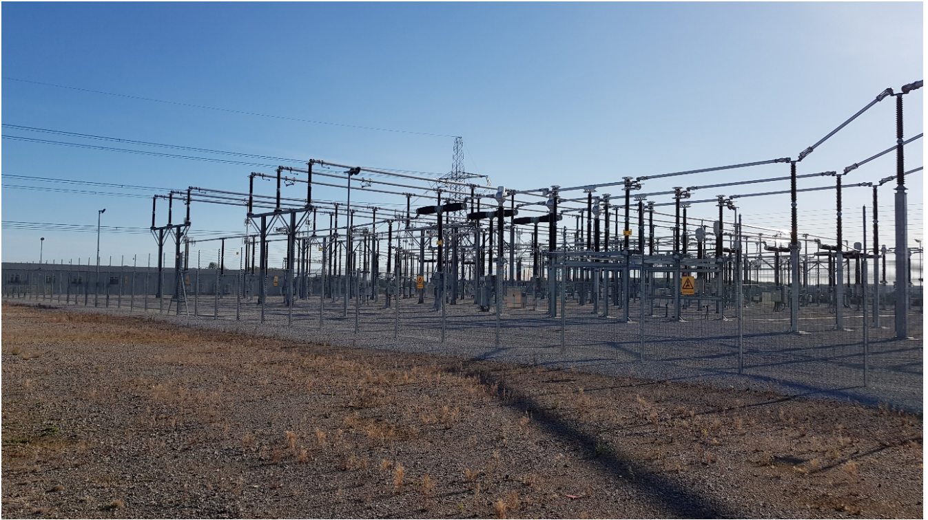
Photograph of proposed fencing at the onshore project substation, taken at the existing Necton National Grid substation, showing 2.4m palisade fence with the further 1.0m electrical pulse fencing mounted upon the palisade fence (Source: GHD).
